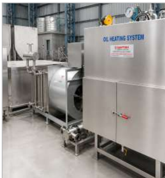
Inline Oil Heating System
